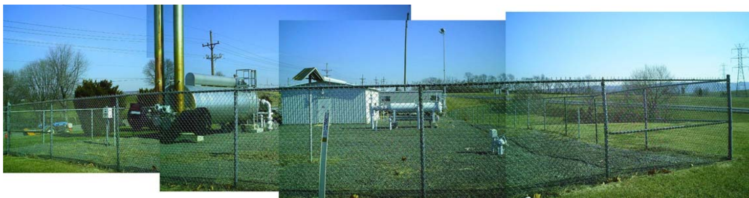
Jefferson Existing Dominion Gas Facility looking East.
